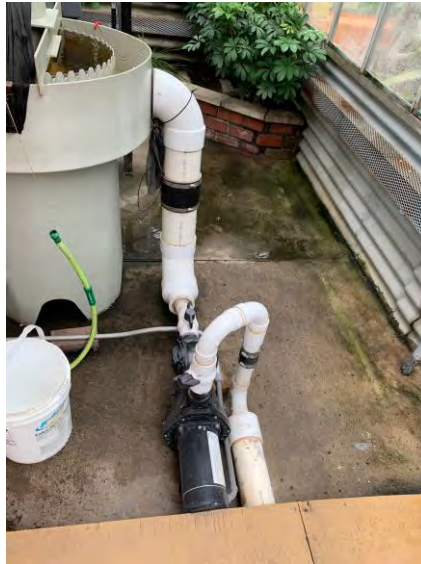
An Example Pipe Set-up from Site Visit
