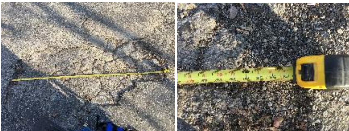
Figures: Measurement of the pothole
