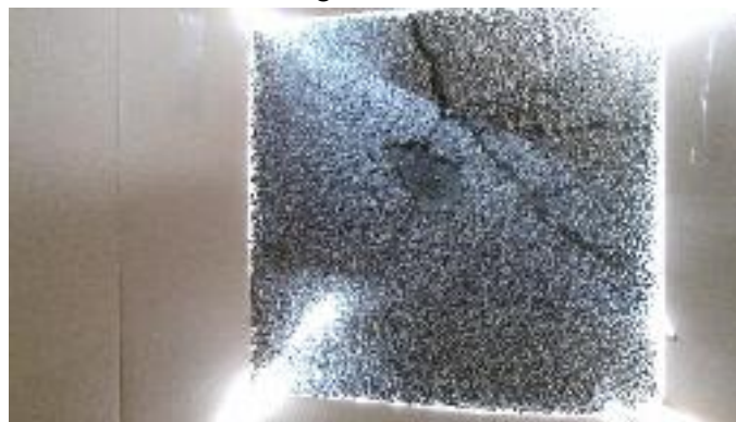
Figure: RGB image for pothole detection test
